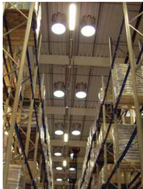
magazzino, Lightway® Silver 600
