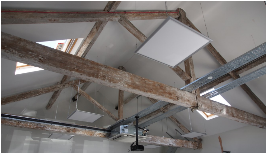
Exposed Mechanical and Electrical Strategy
